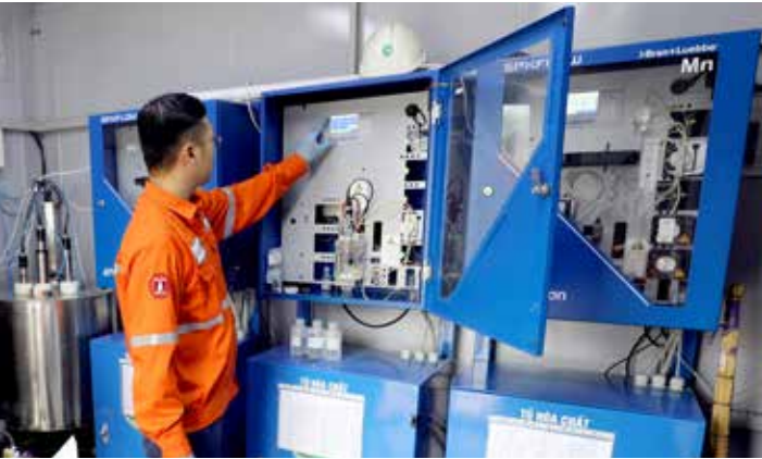
Automatic wastewater monitoring station at NPMC
