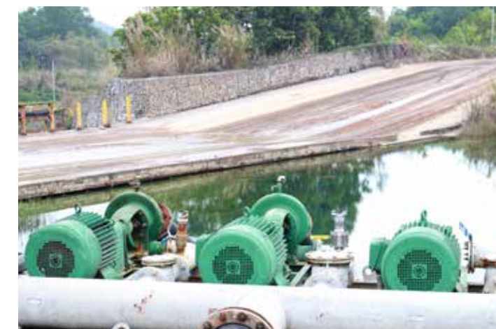
Emergency pumps at TSF-SP pond
