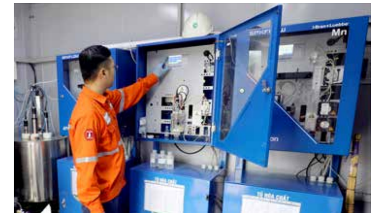
Automatic wastewater monitoring station at NPMC
