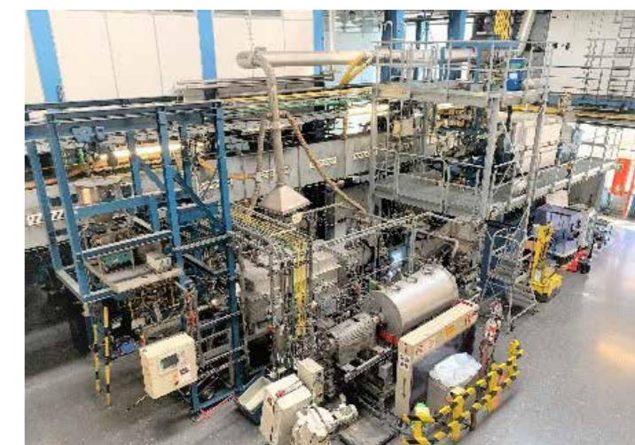
HCS Technology & Innovation Global - High Temperature Pilot Plant (Goslar, Germany)
