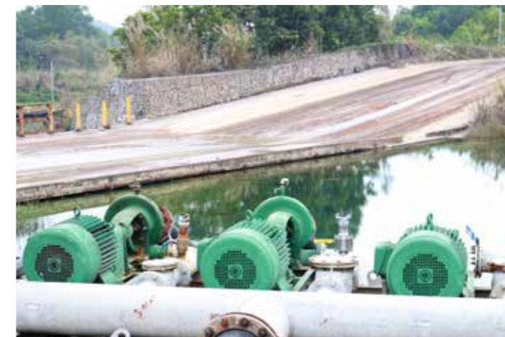
Emergency pumps at TSF-SP pond
