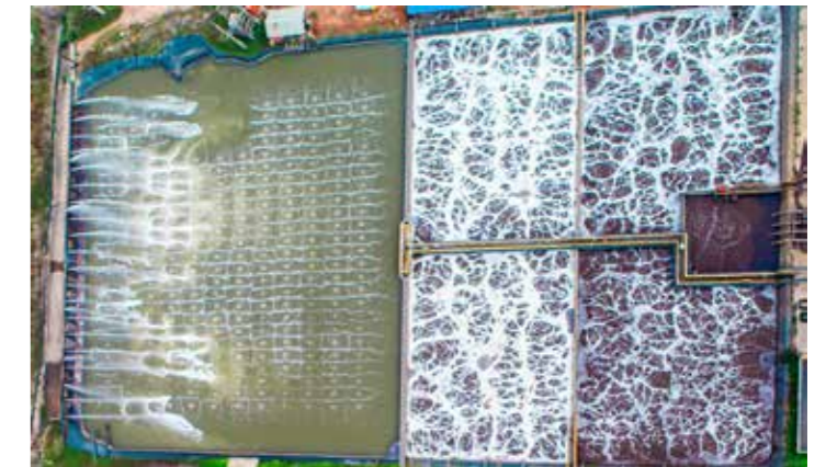
A part of MHT waste water treatment plant in Vietnam
